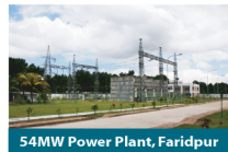
54MW Power Plant, Faridpur
