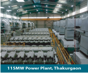
115MW Power Plant, Thakurgaon
