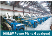
108MW Power Plant, Gopalganj
