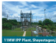
11MW IPP Plant, Shayestagonj
