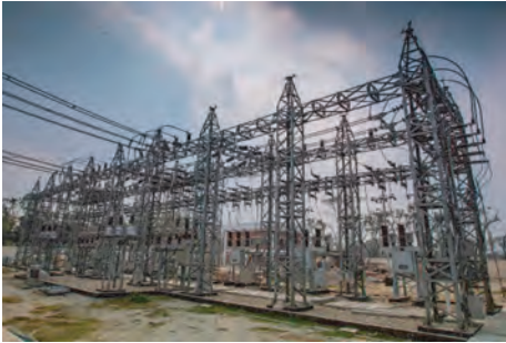
230/33KV, 120/140MVA GIS Substation at Mirsharai EZ and extension of 230 kV GIS bays at existing of 230/33kV BSRM Substation on Turnkey Basis owned by PGCB.
