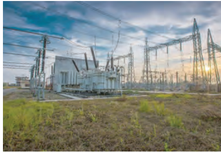
Scope of the Project was EPC of 230kV and 400kV Switchyard for Bibiyana III 400MW CCPP owned by Larsen & Toubro Limited
