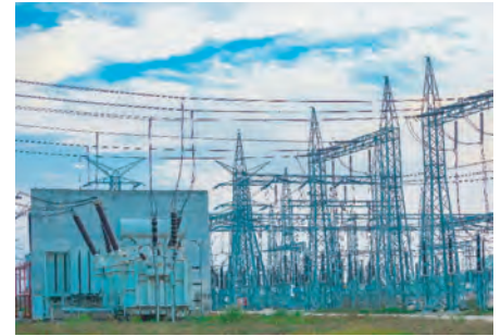
Design, Supply, Testing & Commissioning work of Bibiyana II 400/230/33KV A15 switchyard owned by Summit Bibiyana II Power Company Ltd.
